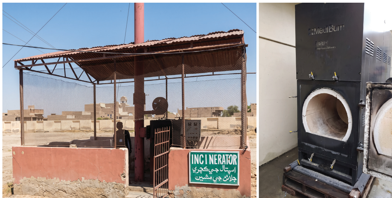
Figure 6-2. Incineration Facilities for Waste Treatment (Pakistan)
